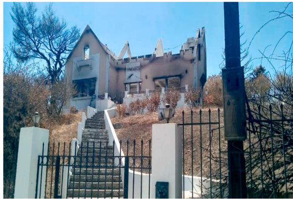
Fig. 5. Building with reinforced concrete frame totally burned after the collapse of the wooden part of the tiled roof, several hours after the fire front had passed.
